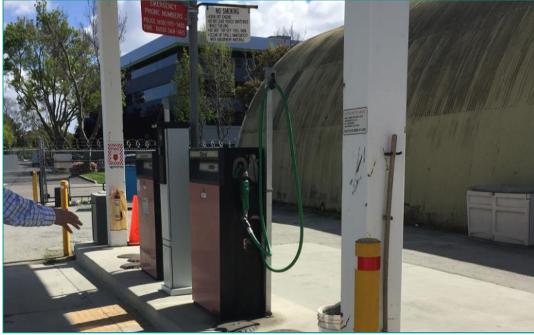
Fuel pumping station at Belmont Corporation Yard.
