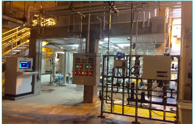
Essential pump control station is underground.
