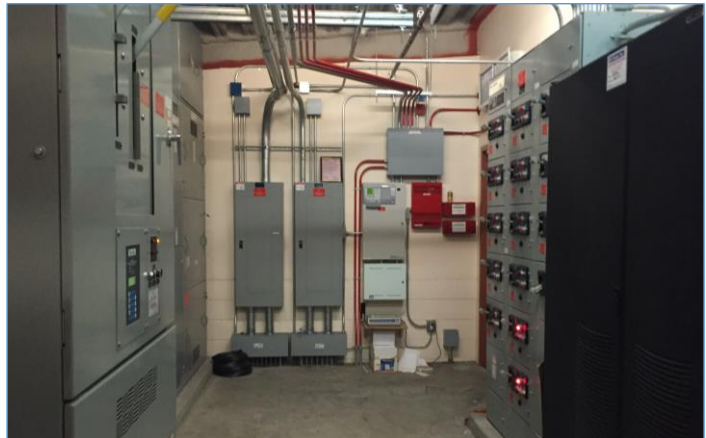
Power systems in the basement of the station.
