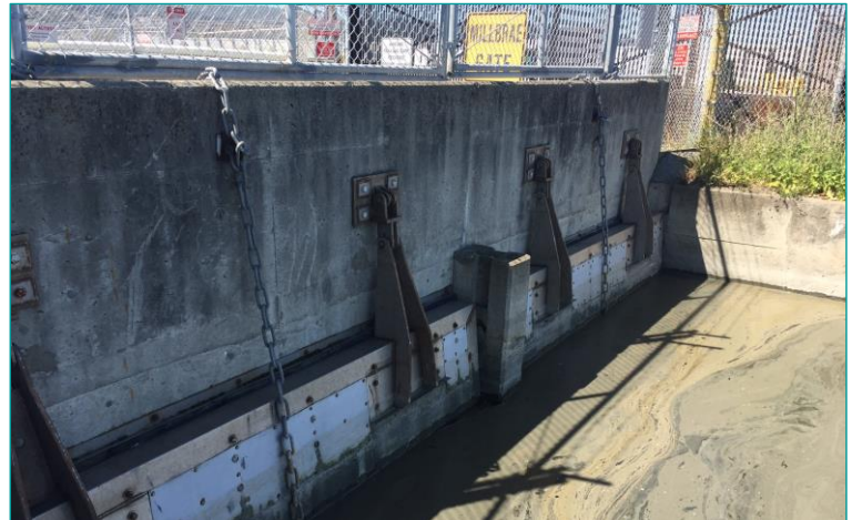
Highline Canal Tide Gates.
