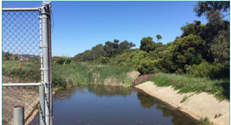
Location where vegetation is growing into concrete channel.
