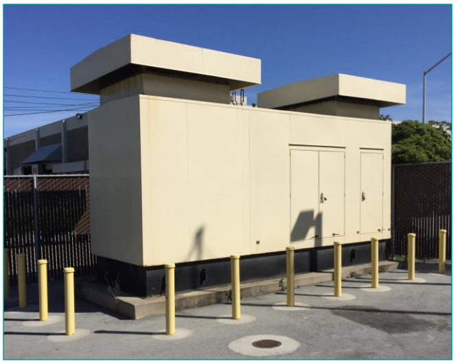
Power distribution system.
